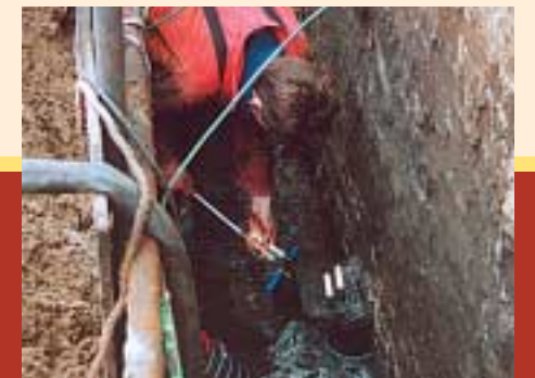
Foundation inspection pit in Haarlem (the Netherlands), piles are measured and sampled.
